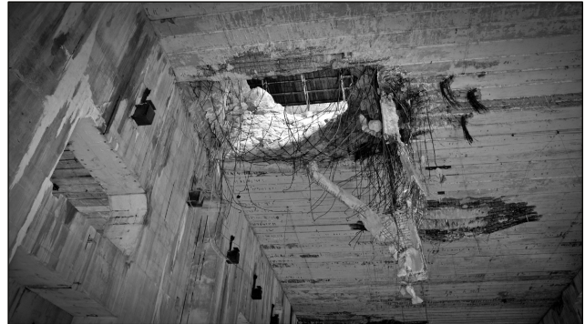
Cracked ceiling of a Soviet Union bunker. (Symbolic image) 26
